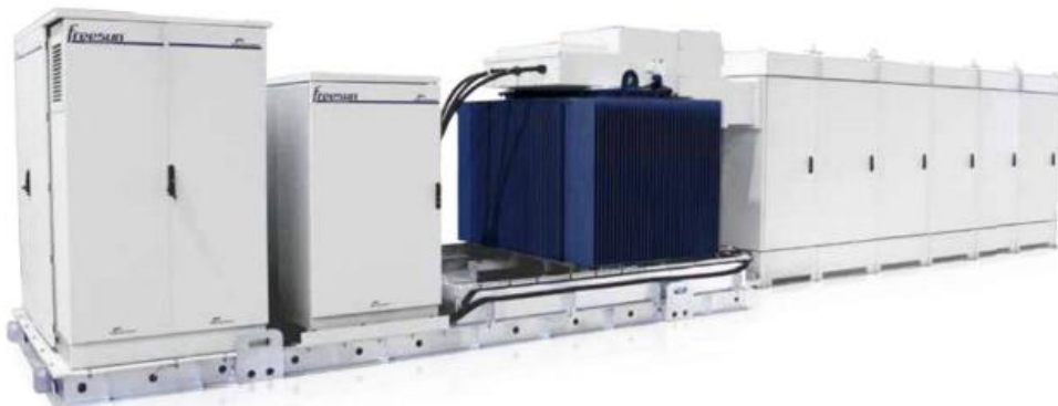
Figura 4. Freesun MV SKID Frame 2.
